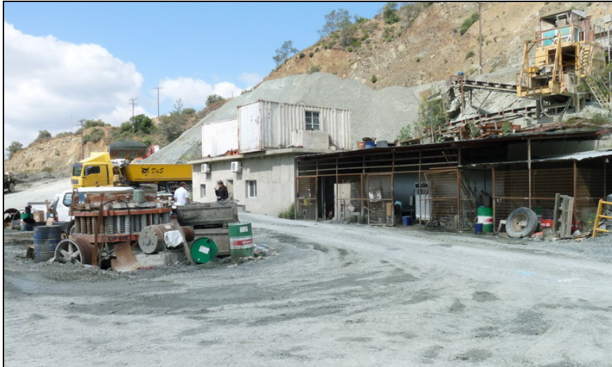
Figure 3 – ZYGOS : Petrol tank (right) and mechanical maintenance zone (left) in solid rock quarry close to Limnatis river.
