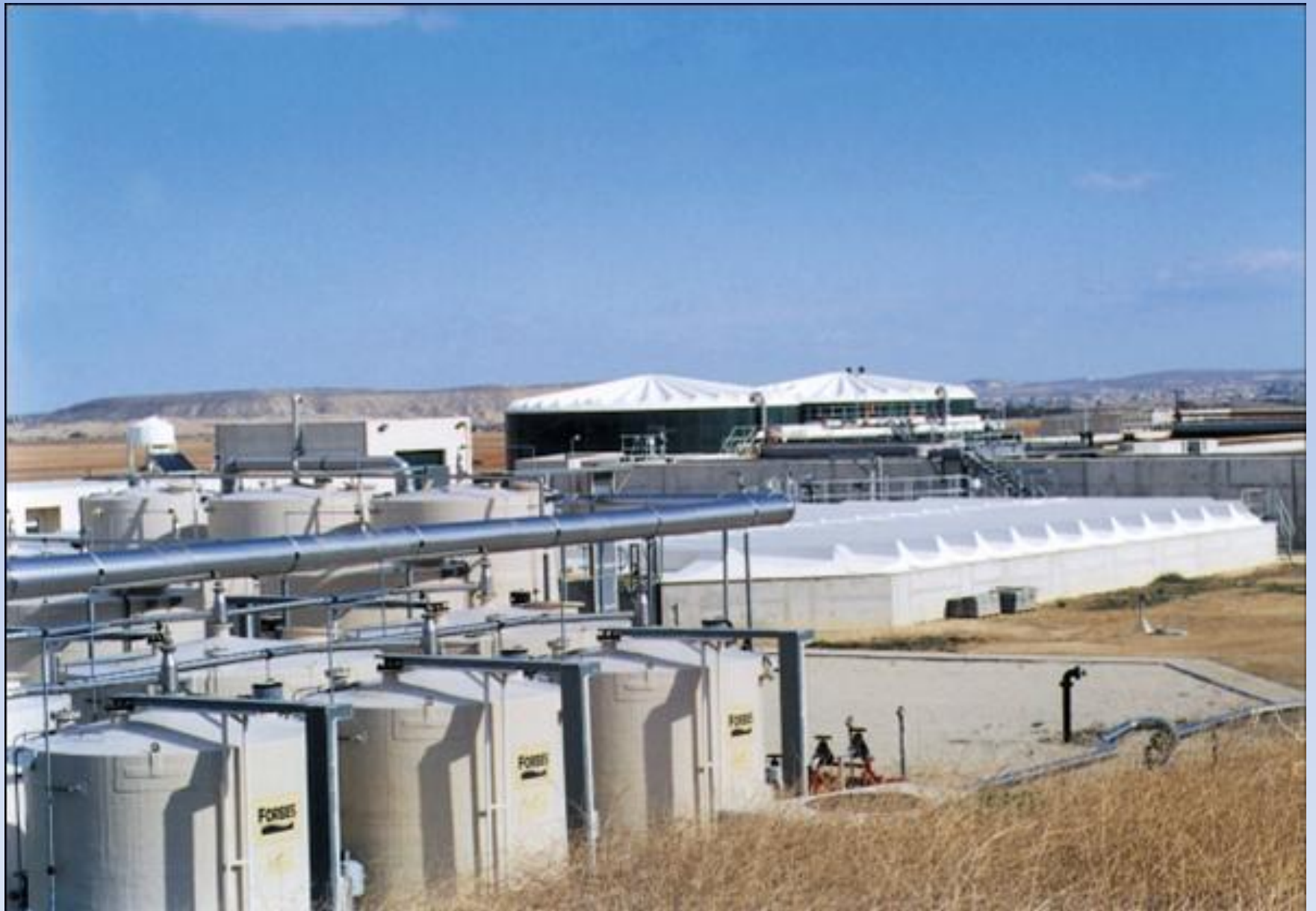
VATHIA GONIA CENTRAL WASTEWATER (SEPTIC SEWAGE/INDUSTRIAL WASTE) TREATMENT PLANT, WDD - 1,320 m 3 /day
